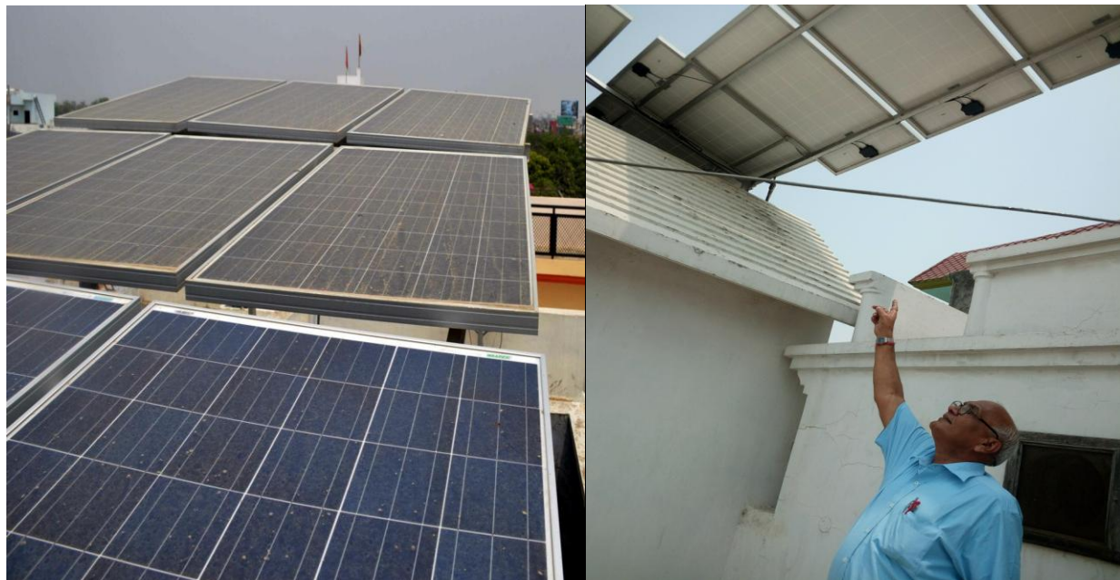
Figure 4: 5-Kw Roof Top Solar PV Plates Installed at Gomati Nagar, Lucknow
