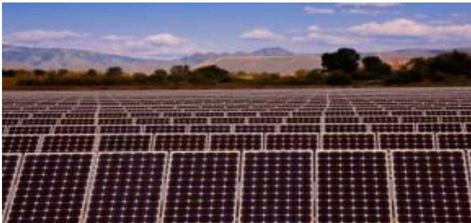
Figure 2: Solar Generation Unit
