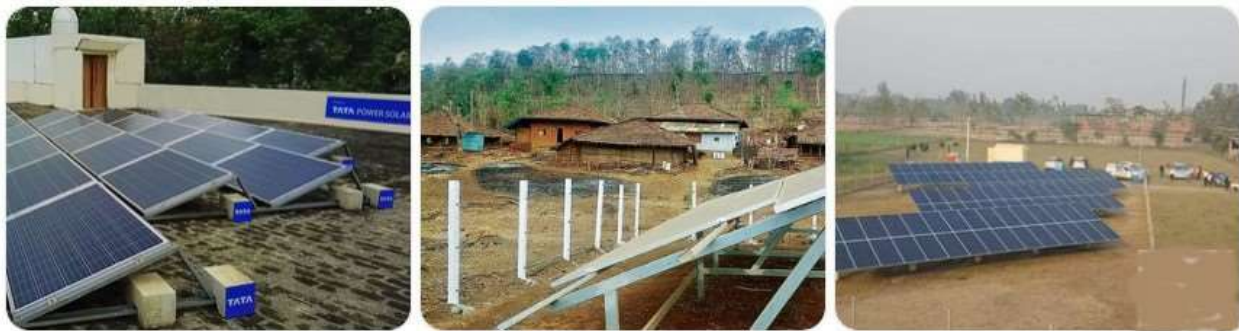
Fig. 7: Indian Rural Micro-Grid – Electrification
